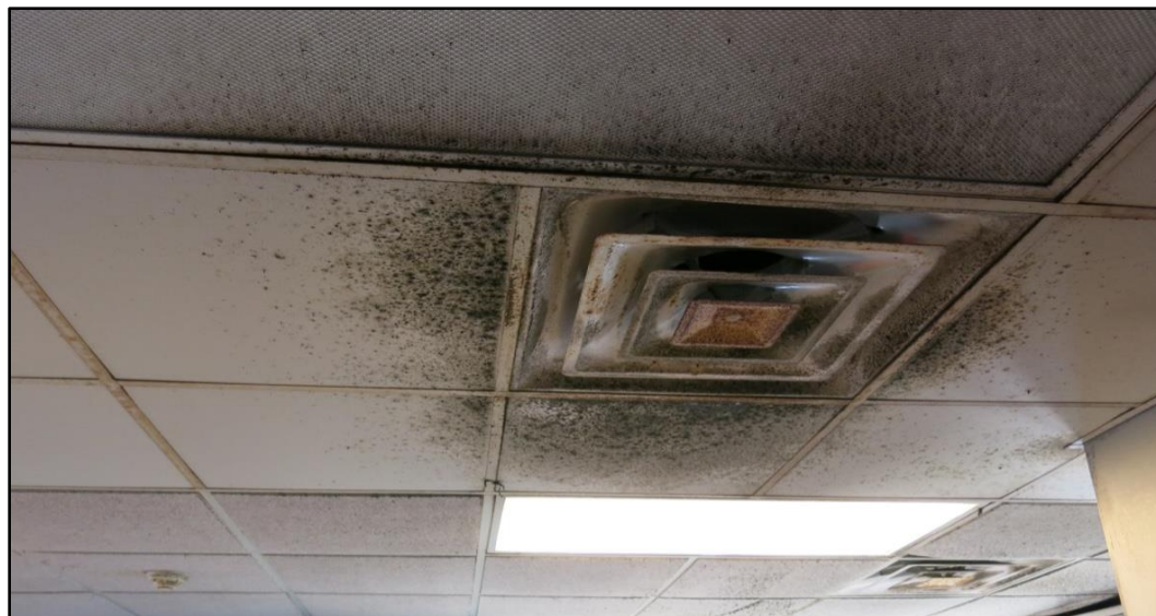
Figure 19. Mold growing near duct vents in Building 2261
