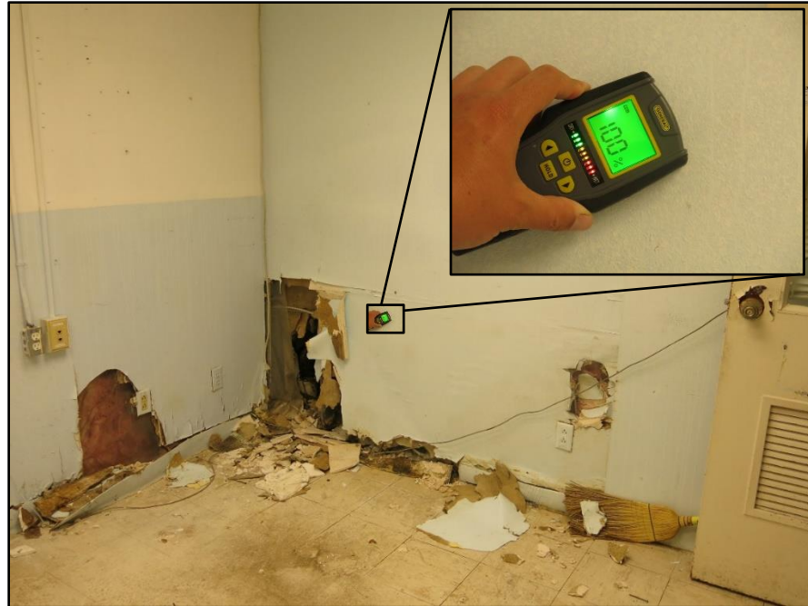
Figure 27. Wall surface moisture content of 100% near sample location #4.
