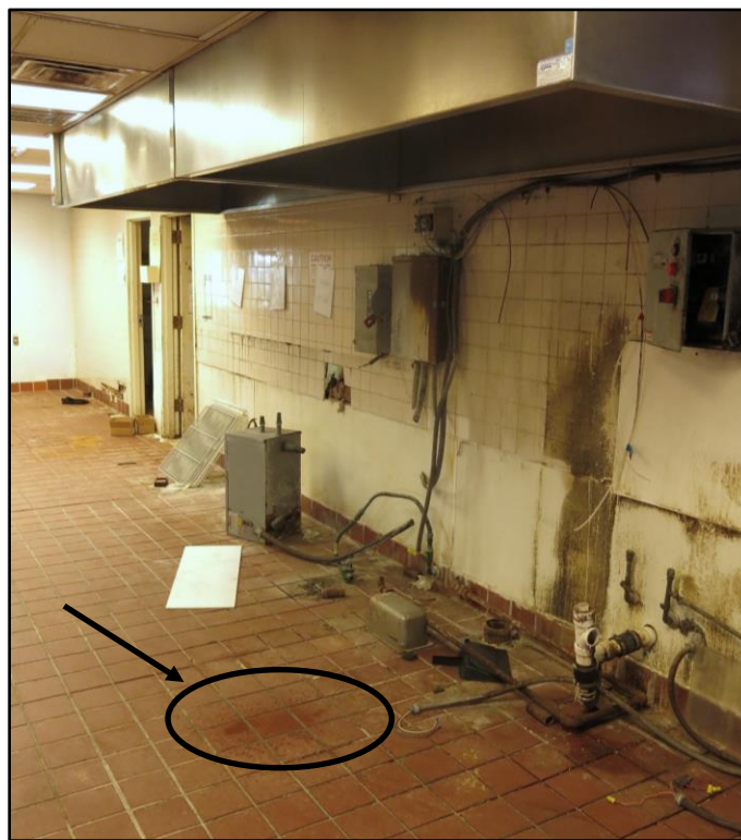
Figure 28. Leakage from ceiling piping or roofing
