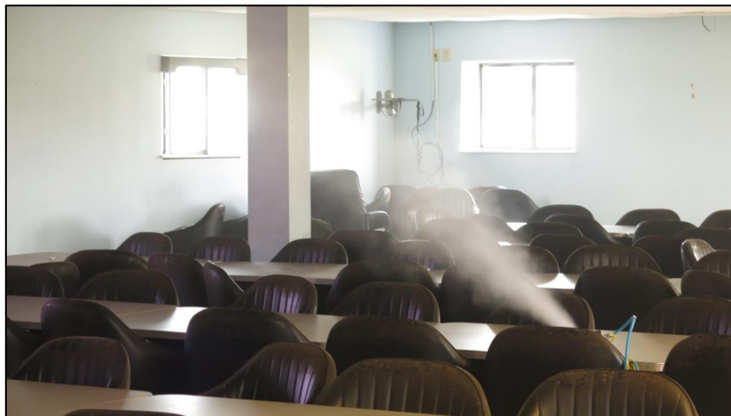
Figure 13. Dry-fog being applied via spray nozzle in Building 2261.
